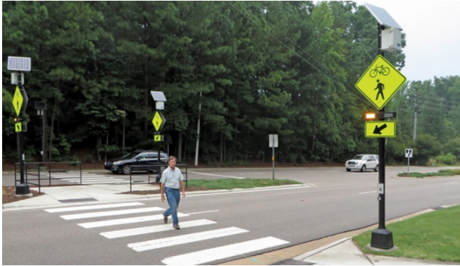
Photo of Rectangular Rapid Flashing Beacon (RRFB) treatment.
